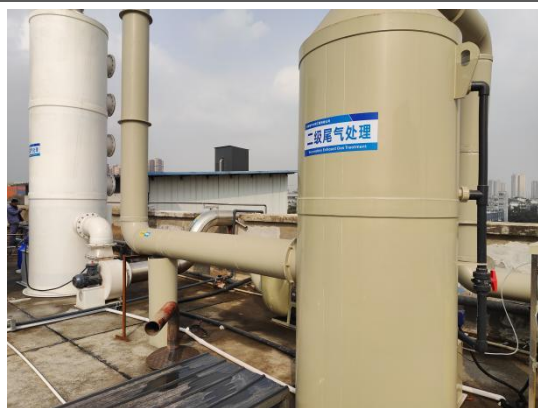
酸洗喷淋+碱洗喷淋
